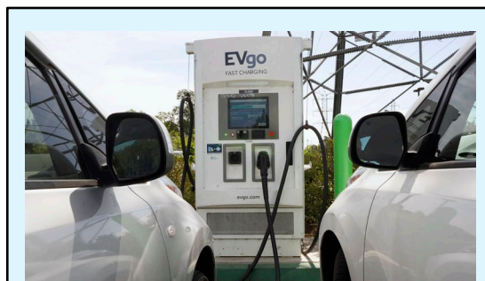
EV charging infrastructure such as this EVgo DC Fast charger are widely available in SCAG region. Around 3,712 DCFC currently are available in SCAG region provided by 20-30 manufacturers.
